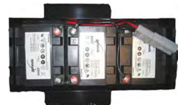
3x42Ah Batteries in series
