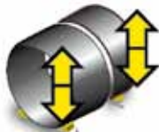
Joining of shell sections using roller beds with hydraulic fit-up system. Internal and external submerged-arc welding performed by a column and boom station.
